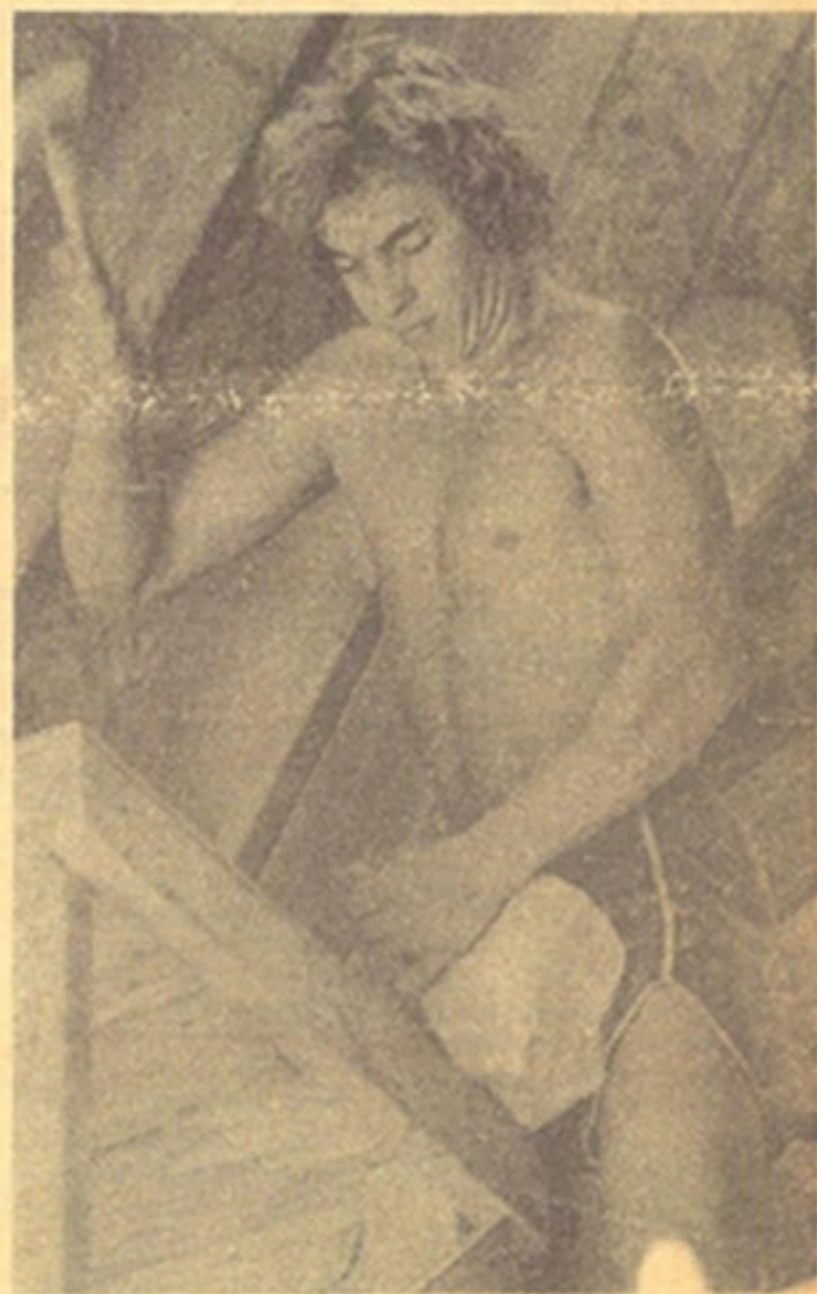
20-year-old John Shell trims one of the few remaining fireplace fieldstones high atop the scaffolding inside the Joseph Duris home.
